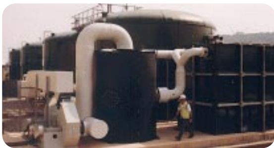
MÓNASHELL Biofilter at Minehead
